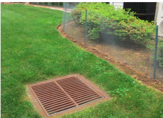
Fig. 2. Dry well installed to receive runoff flowing through a lawn (Source: R. Pitt)
