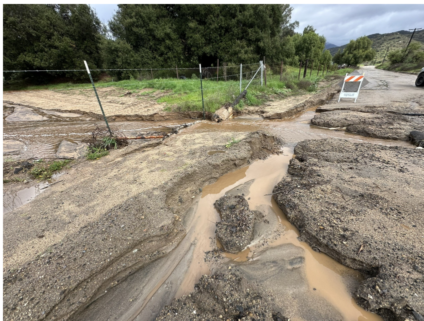
Figure 6.7.8. Flood Damage on Lilac Road in Pala, February 2024.
