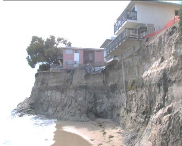
Figure 4. Cliff collapse at Isla Vista, California (taken 2005)
