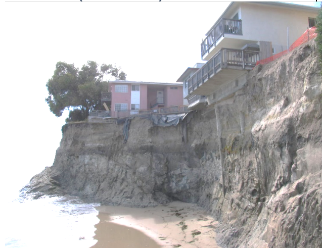
Figure 4. Cliff collapse at Isla Vista, California (taken 2005)
